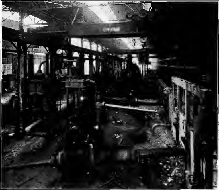
FIG. 97.—Fuller No. 201, 10 furnaces, 5 Boilers.
